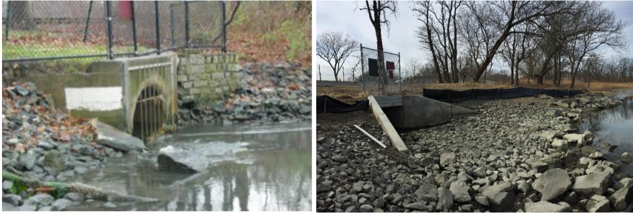
Figure 11. Example of an undersized culvert (left) in 2013 into Eastchester Bay and following replacement (right) in 2016 at Turtle Cove in Pelham Bay Park, Bronx.
