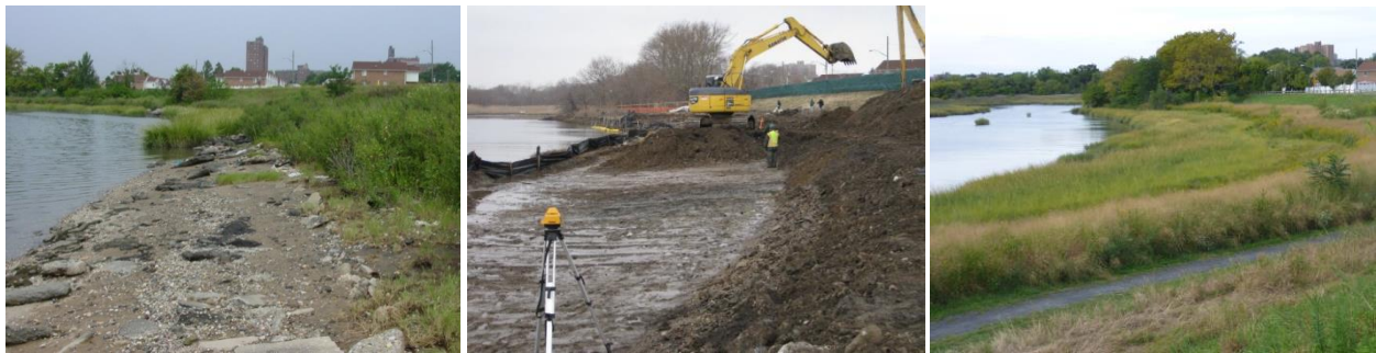
Figure 15. Salt marsh restoration involving over-excavation of fill and placement of clean substrate at Pugsley Creek in The Bronx, NY Images show the site before, ca. 2008 (left), during, ca. March 2011 (middle), and after restoration, ca. September 2015 (right).
