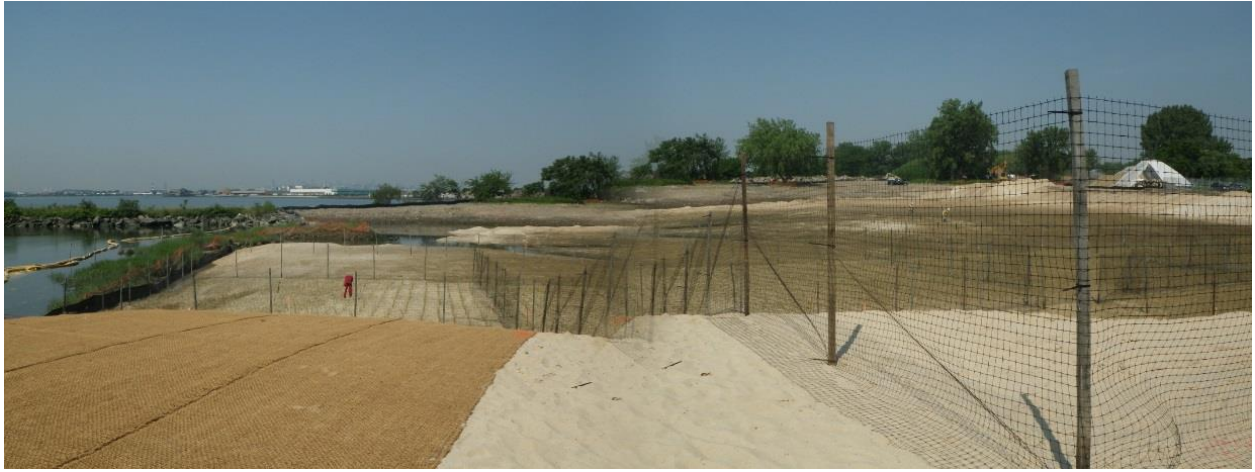
Figure 20: Example of coir webbing installed on upland slope at Soundview Park, Bronx.
