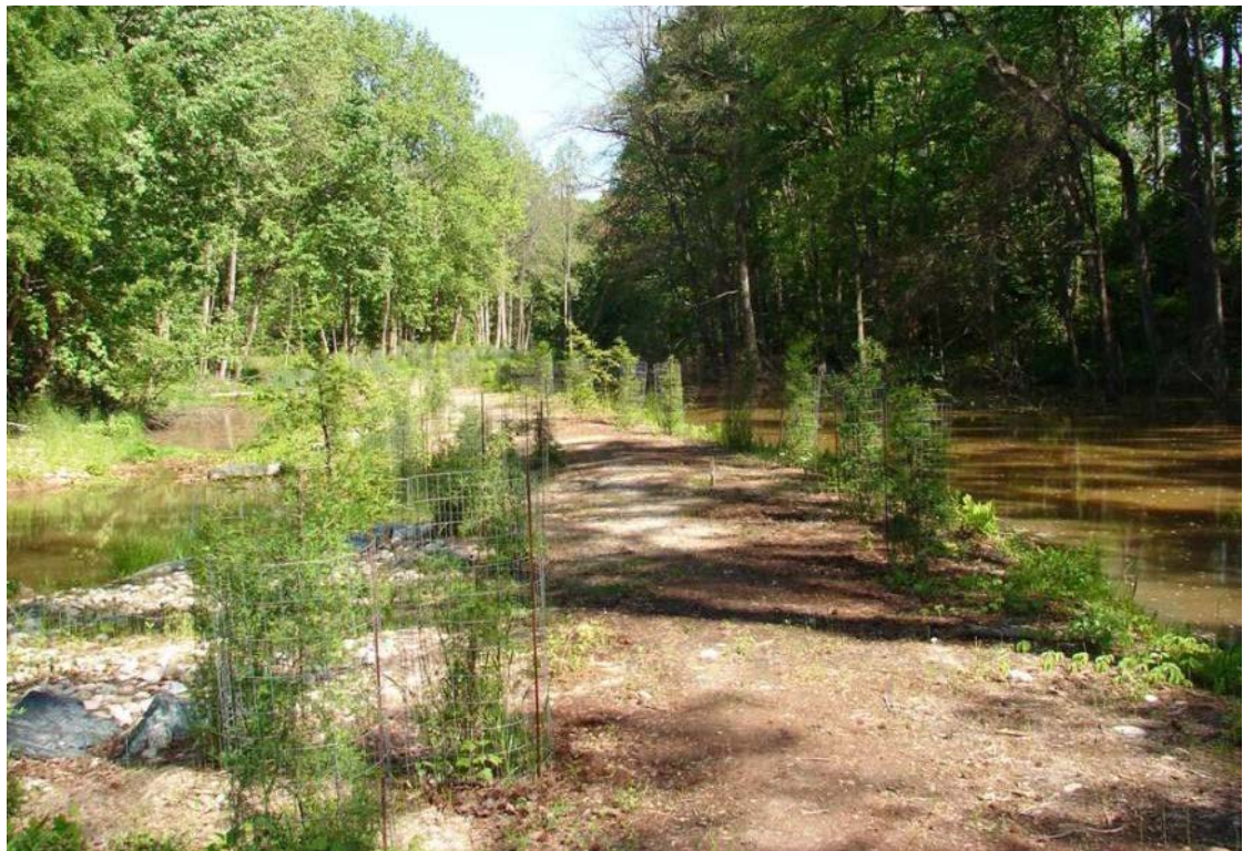
Sand seepage berm constructed as part of the Lizard Hill Wetland Restoration in Worcester County, Maryland.
