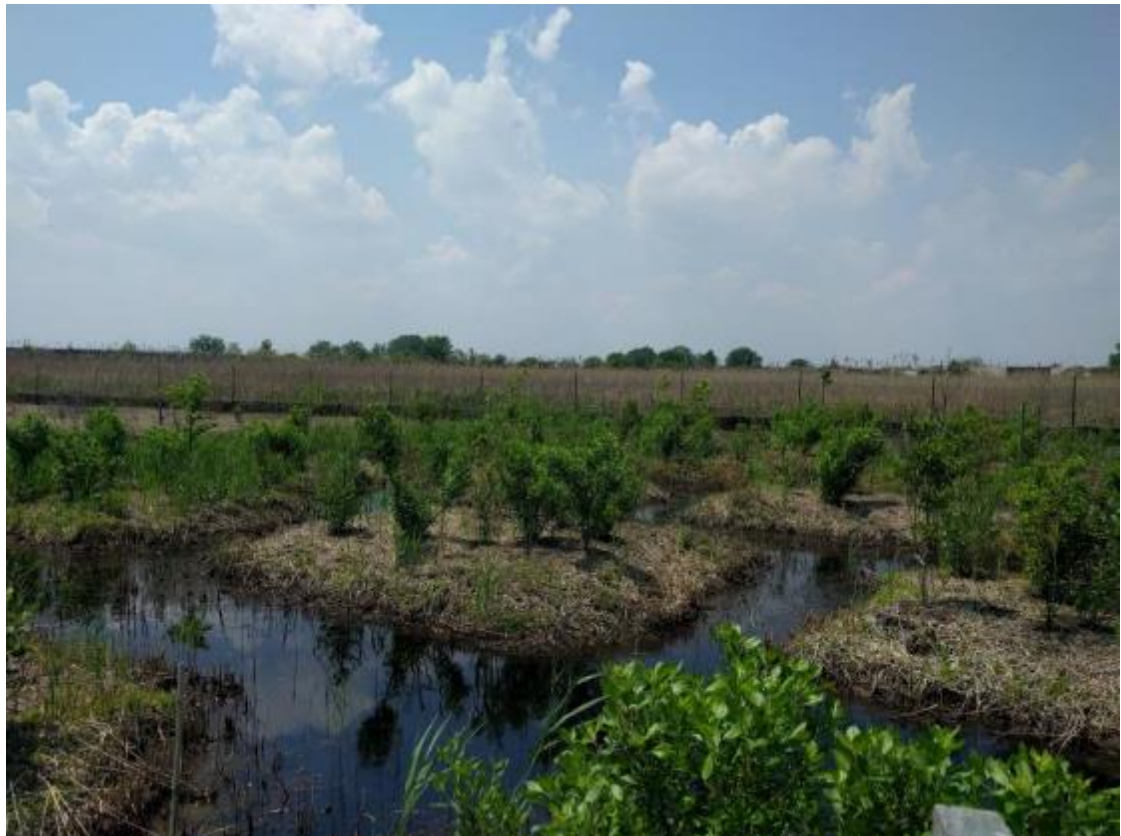
Microtopographic grading and wetland plantings constructed at a Port Authority of New York and New Jersey site.
