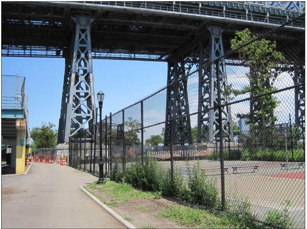
Williamsburg Bridge (#2). View north within East River Park adjacent to FDR Drive 4
