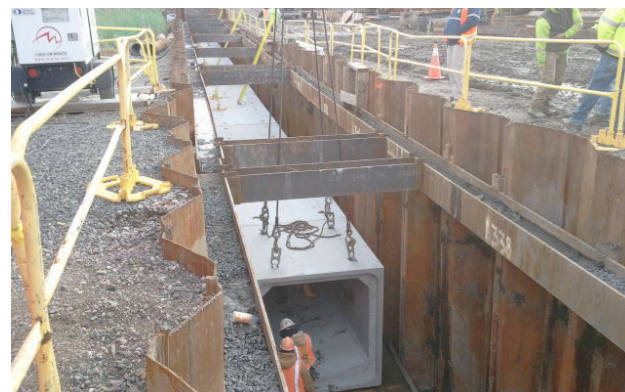
From top: Large-scale subsurface detention crates can store volumes of stormwater; high-capacity, large-scale interceptors can store and convey large volumes of rainfall and connecting outfalls. Interceptors can connect centralized and decentralized measures.
