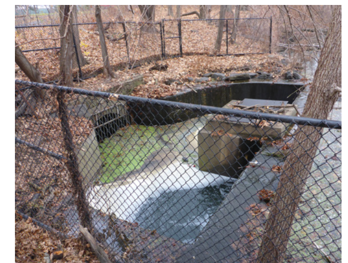
Van Cortlandt Lake weir and outlet where water is then piped into the combined sewer system.
