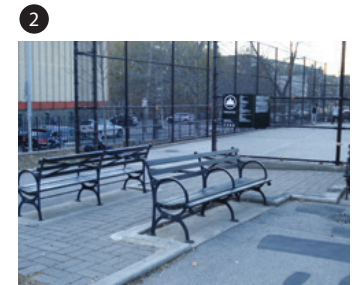
Low point in seating area.
