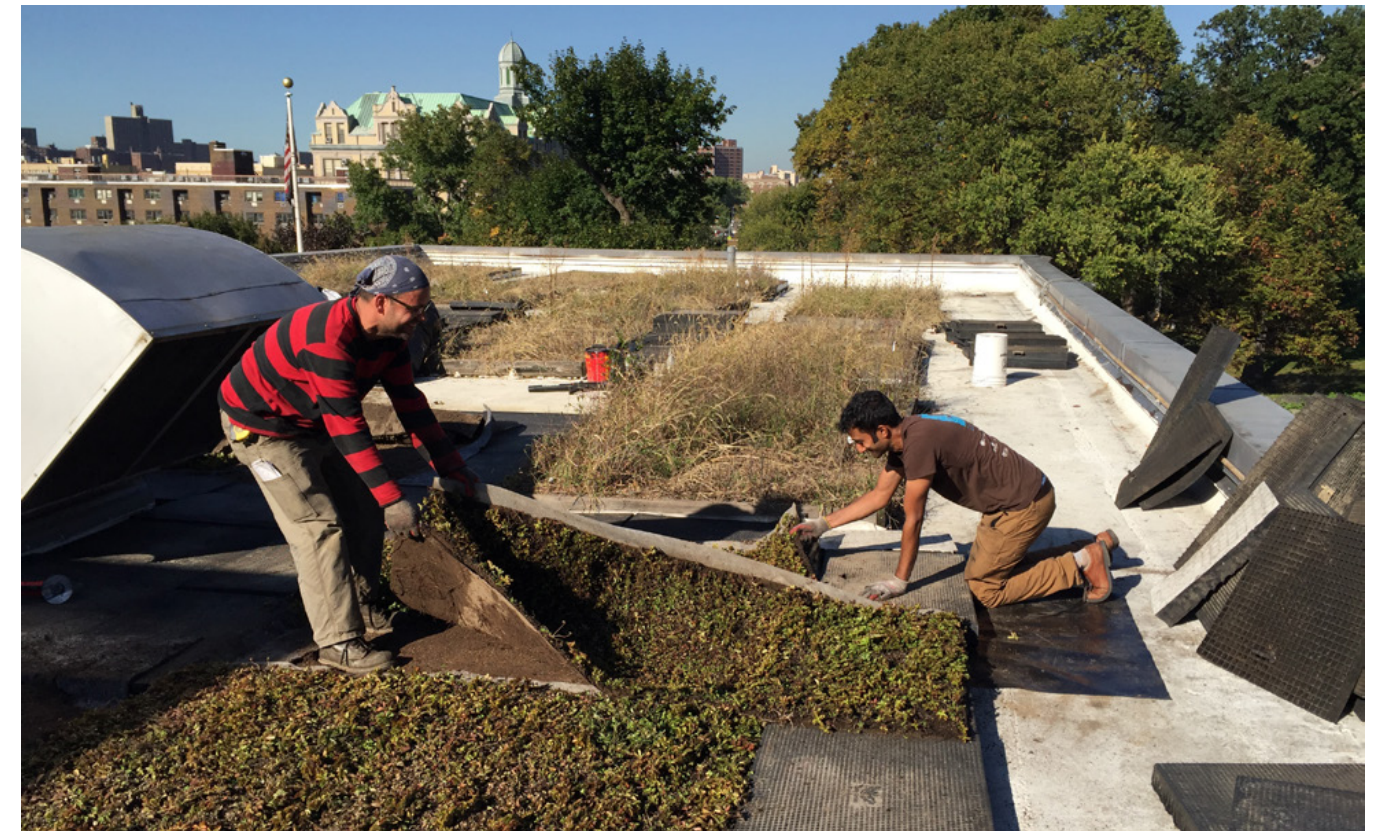
NYC Parks staff install a green roof on the Ranaqua office, Bronx.
