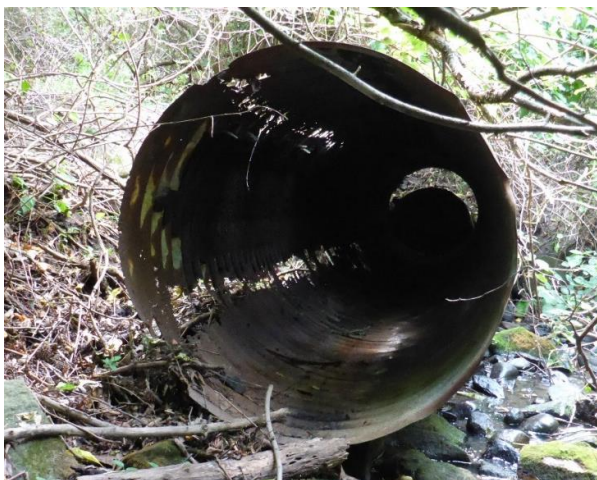
c) Broken culvert at LaTourette
