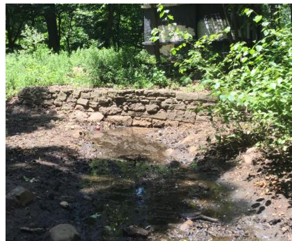
b) Blocked culvert in Van Cortlandt
