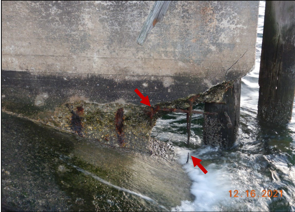
Photo 3.2-21. Severe spall 4 ft long by 2.5 ft high by 10 in. deep in the concrete ramp wall at the Coal Pier with exposed corroded steel reinforcement up to 100 percent, looking east.
