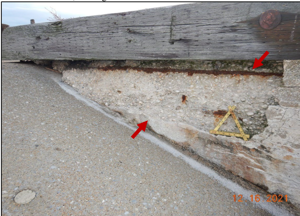
Photo 3.2-20. Severe spall 6 ft long by 3 ft high by 3 in. deep in the concrete ramp wall at the Coal Pier with exposed corroded steel reinforcement up to 30 percent, looking east.
