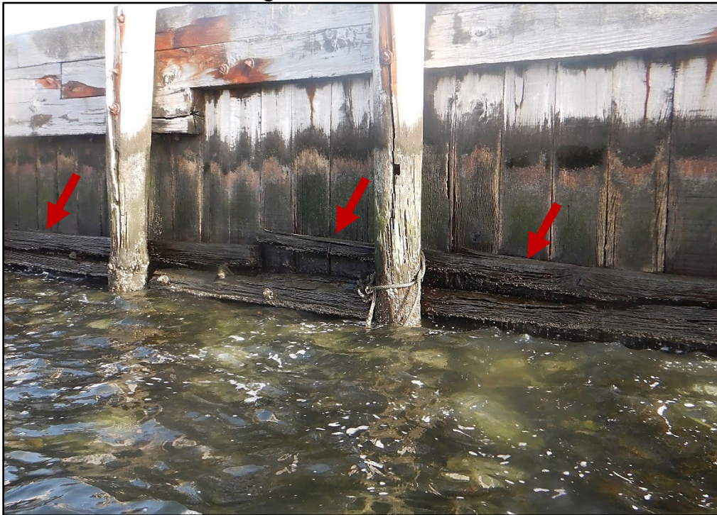
Photo 3.1-6. Low-water timber wale at the Hart Island Ferry Dock Shoreline exhibiting severe splitting and deterioration due to marine borers, looking east.
