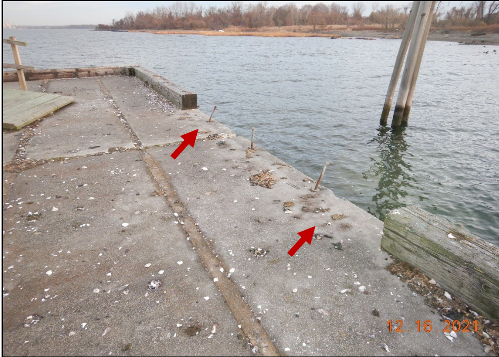
Photo 3.2-23. Missing section of curb up to 15 ft atop the south section of the main loading platform of the Coal Pier, looking north.
