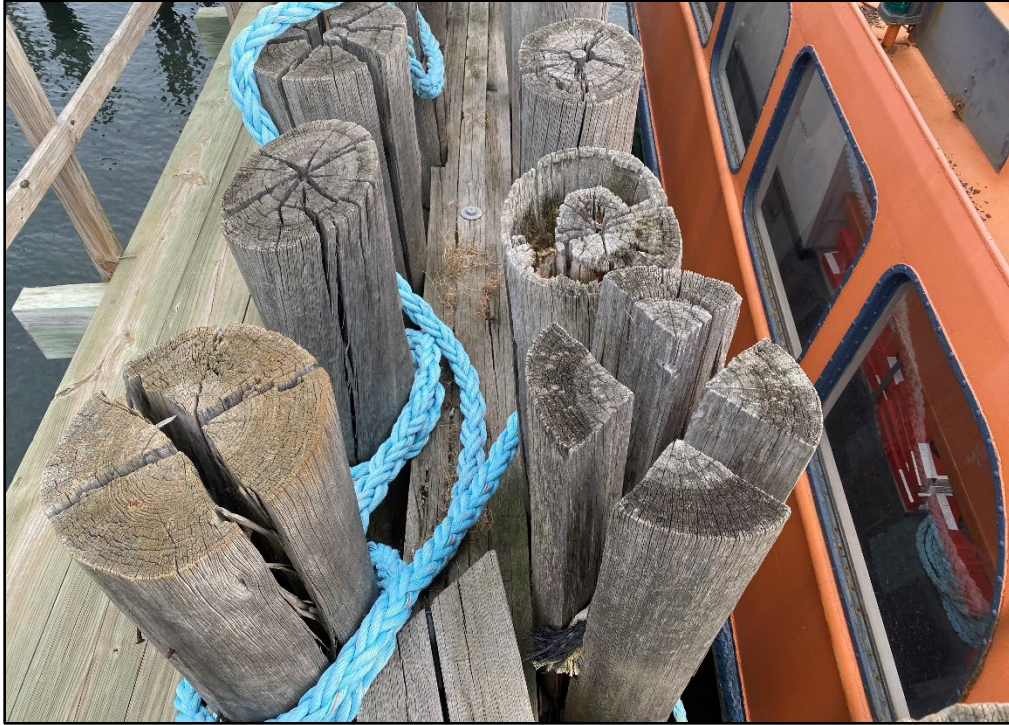
Photo 3.2-5. Tops of the timber piles making up the south timber fender rack at City Island with splitting and hollowing due to rotting, looking east.
