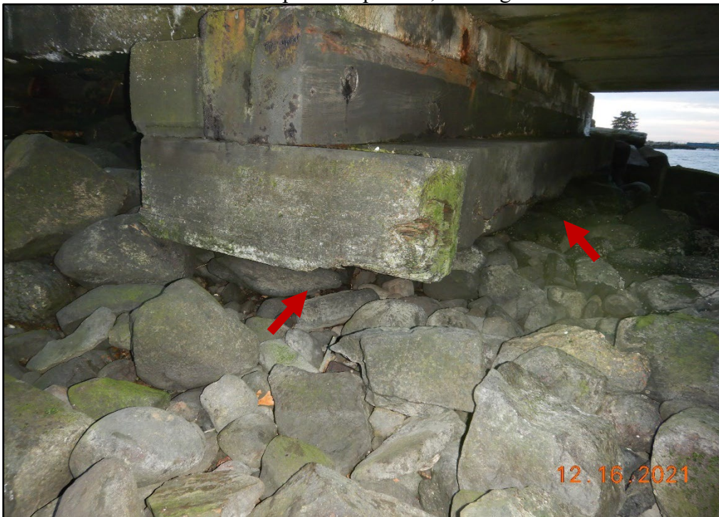
Photo 3.2-22. Undermining more than 3 ft deep beneath the concrete abutment supporting the Coal Pier, looking south.
