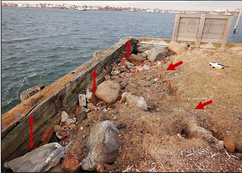
Photo 3.1-3. Subsidence areas behind timber bulkhead at the Hart Island Ferry Dock Shoreline with varying stages of repair fills due to active fill loss, looking west.
