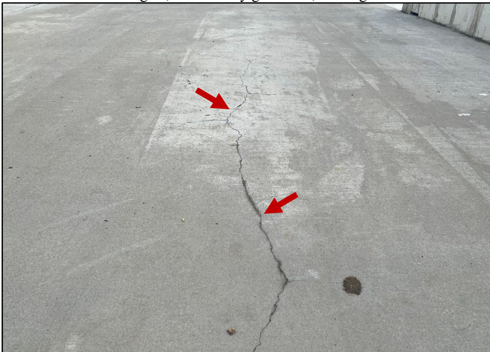
Photo 3.2-2. Minor cracking up to 1/16 in. wide on the concrete deck of the newly constructed Fordham Street Pier, looking west.
