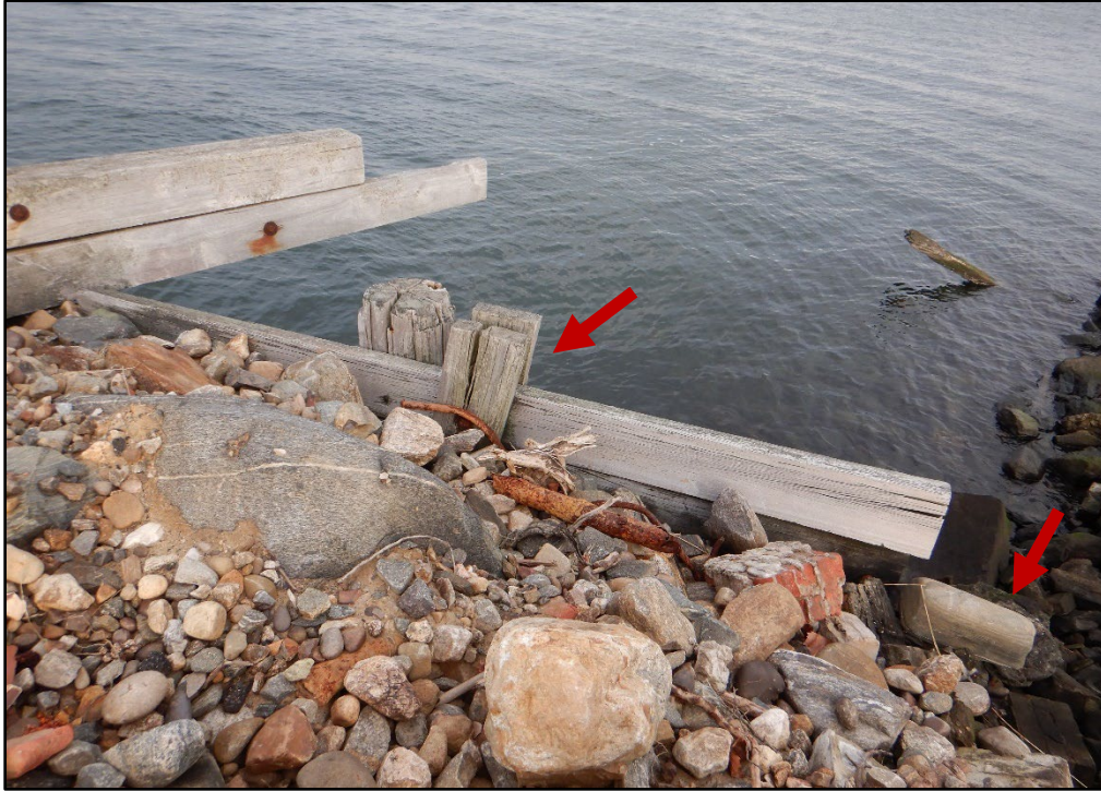
Photo 3.1-7. Missing top horizontal timber sheet at the end section of timber bulkhead at the Hart Island Ferry Dock Shoreline with signs of active fill loss, looking north.
