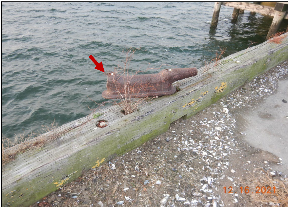
Photo 3.2-24. Broken and loose steel cleat atop the timber curb at the north side of the landing access platform of the Coal Pier, looking south.
