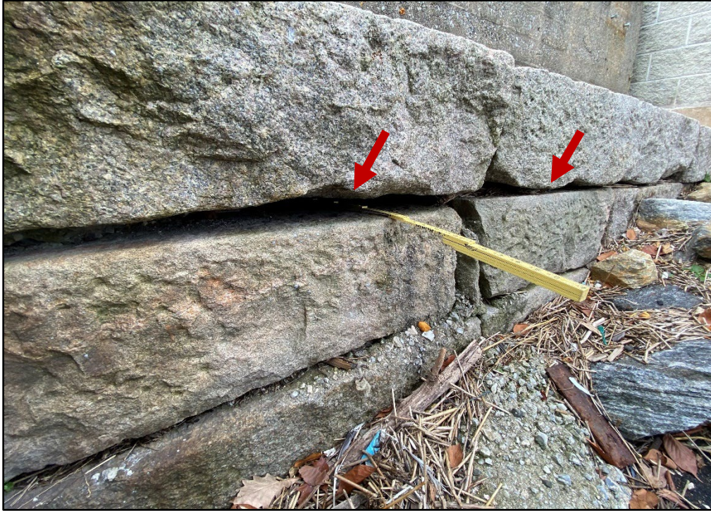
Photo 3.1-1. Masonry bulkhead at the Fordham Street Shoreline with widespread grout loss up to 3.5 ft deep, looking west.
