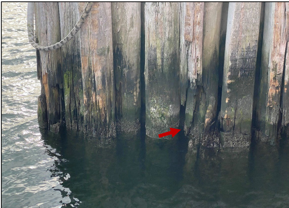
Photo 3.2-4. Broken timber piles comprising the south timber fender rack at City Island, looking south.
