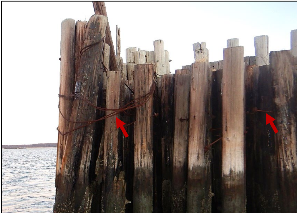
Photo 3.2-12. Loose steel cable wraps and steel connection hardware securing the south timber fender rack at Hart Island, looking north.
