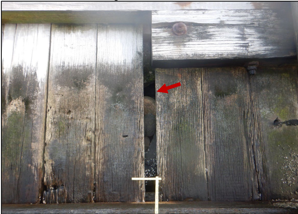
Photo 3.1-4. Timber bulkhead at the Hart Island Ferry Dock Shoreline with gaps between the sheets up to 3.5 in. wide and over 12 in., looking east.
