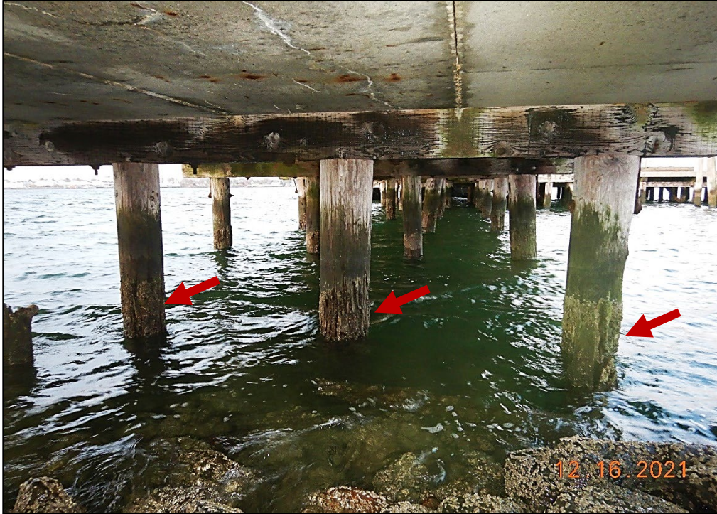
Photo 3.2-15. Timber piles at Bent 1 supporting the Coal Pier with peeling, abrasion, and section loss due to marine borers, looking west.
