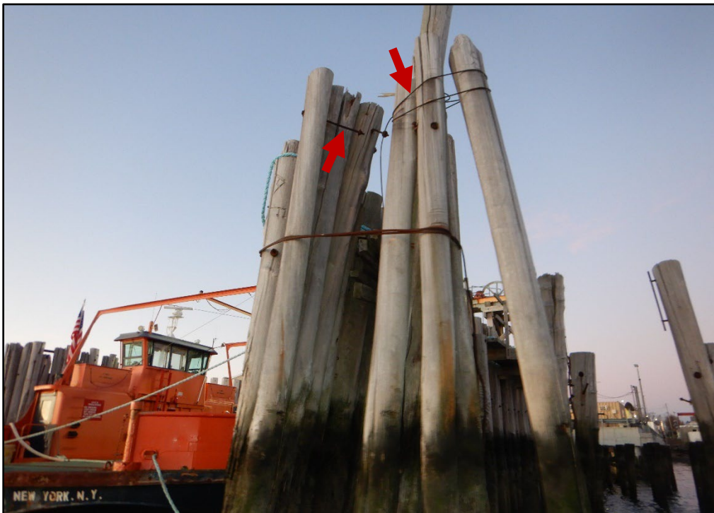
Photo 3.2-6. Loose, missing, and broken steel connection hardware and steel cable wraps with surface corrosion securing the north timber fender rack at City Island, looking east.
