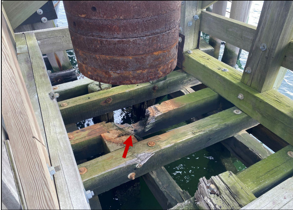
Photo 3.2-7. Broken horizontal posts beneath the steel gantry weights due to impact at the south timber gantry tower at City Island, looking southeast.
