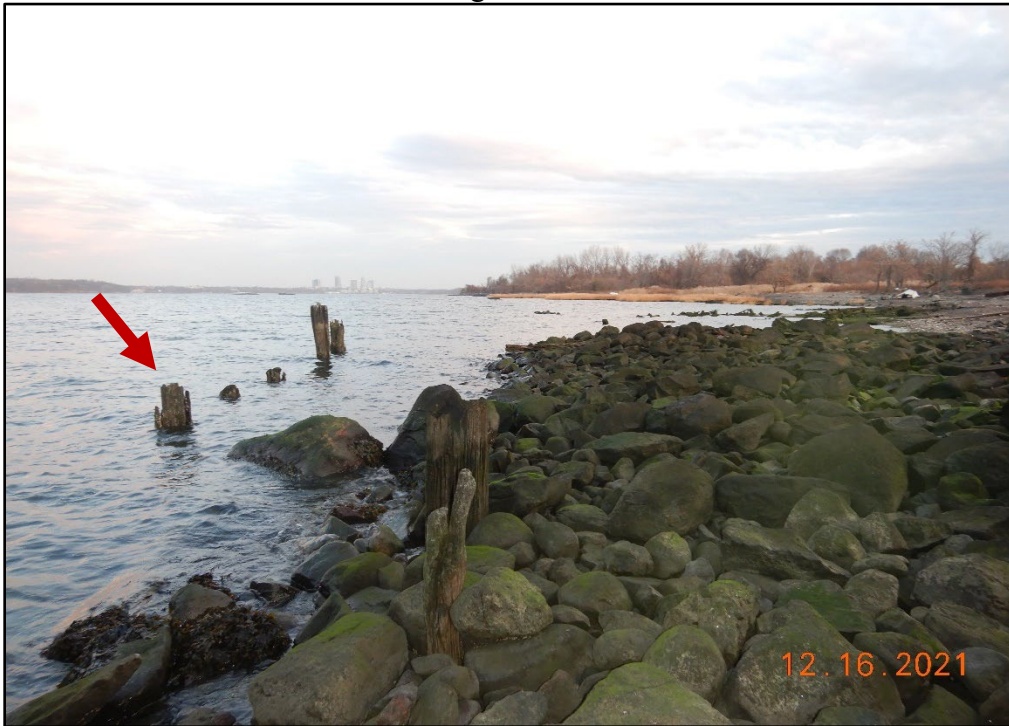
Photo 3.1-8. Poorly graded riprap stone and timber cutoff piles at the Hart Island Coal Pier Shoreline, looking north.
