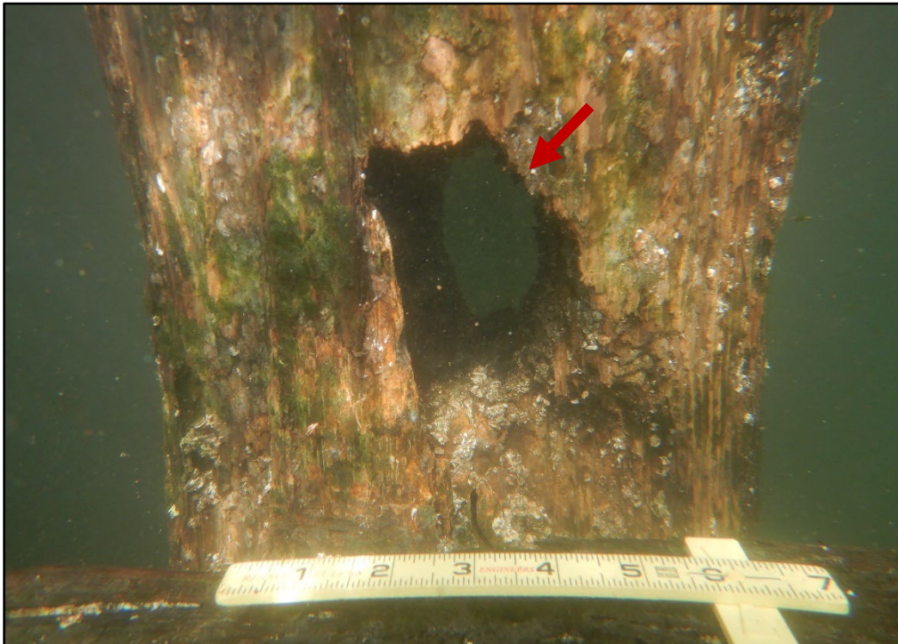
Photo 3.2-16. Timber Pile 9-F supporting the Coal Pier with section loss at a hollowed-out hole due to marine borers, looking north.
