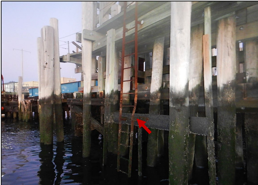
Photo 3.2-8. Safety ladder with impact damage and moderate corrosion at the south timber gantry tower at City Island, looking west.
