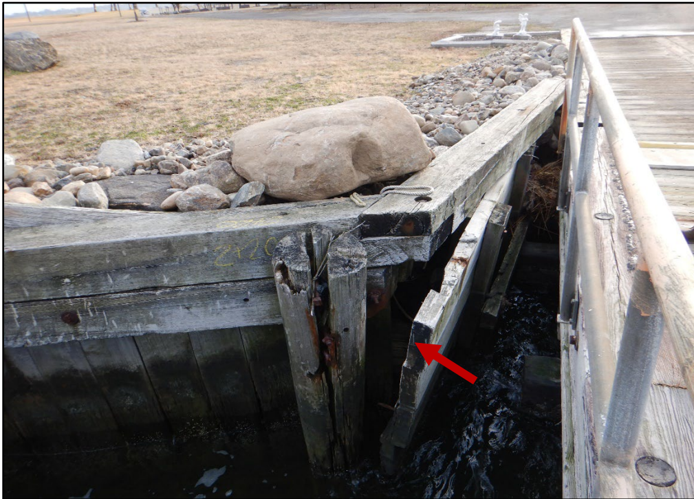
Photo 3.1-2. Timber bulkhead at the Hart Island Ferry Dock Shoreline with gaps up to 8 in. wide and over 12 in. deep with exposed fill within, looking east.
