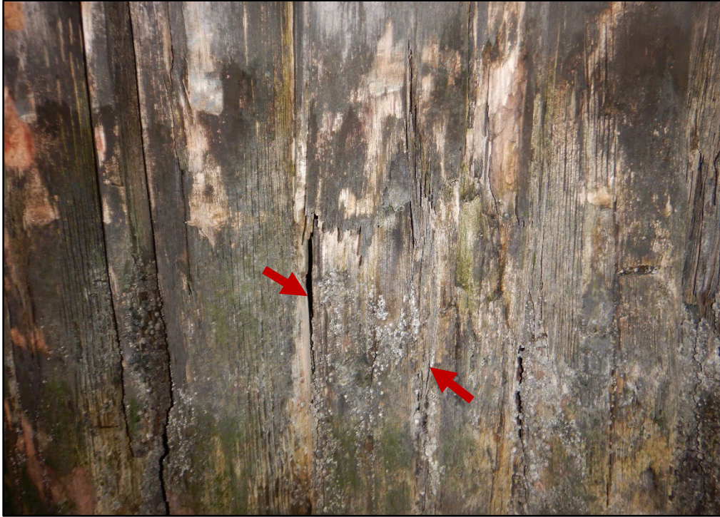
Photo 3.2-3. Timber pile making up the north timber fender rack at City Island with 30 percent section loss, looking northwest.
