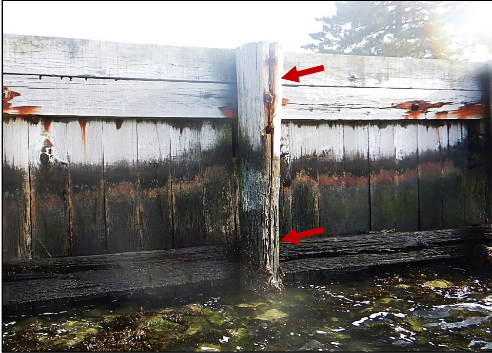
Photo 3.1-5. Timber soldier piles at the Hart Island Ferry Dock Shoreline exhibiting advanced splitting and deterioration due to marine borers, looking east.
