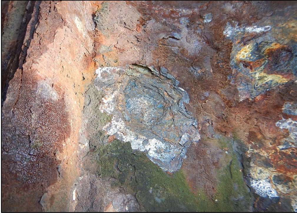
Photo 3.2-13. South steel sheet pile cell supporting the gantry at Hart Island with advanced section loss due to corrosion, looking north.
