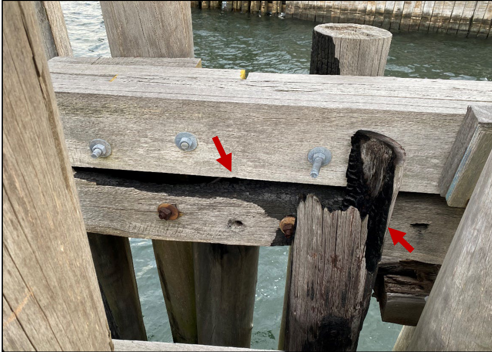
Photo 3.2-11. Horizontal timber posts securing the south timber fender rack at Hart Island exhibiting fire damage, looking north.
