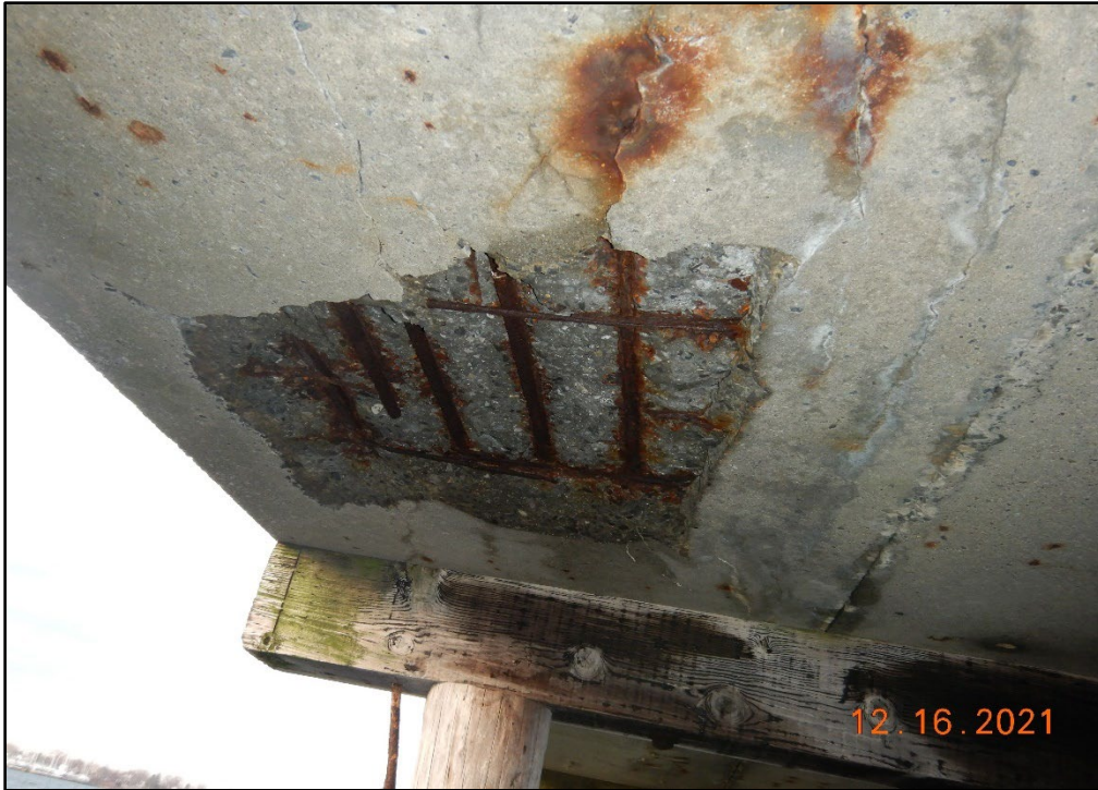
Photo 3.2-19. Severe spall in the precast concrete deck with exposed corroded steel reinforcement up to 100 percent east of Pile 1-A' at the Coal Pier, looking west.
